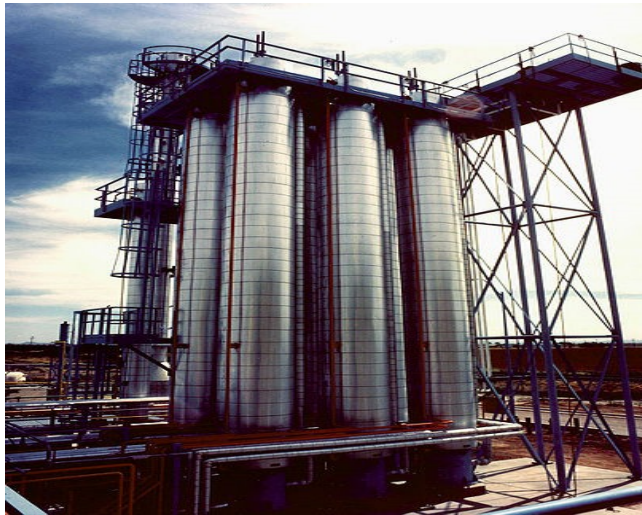
Chemical processing equipment at a P.S.T. poly-silicon plant
