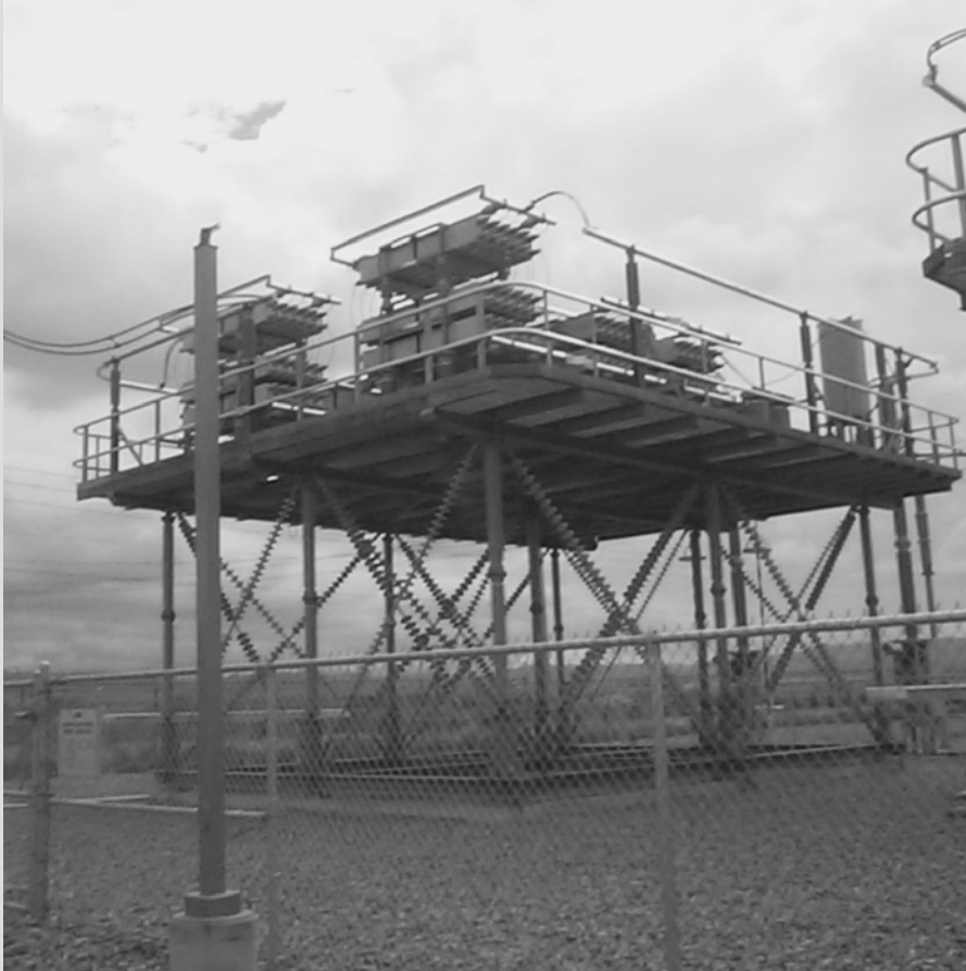
Series capacitor installation at Goshen Substation, Goshen, Idaho, USA rated at 395 kV, 965 Mvar (Courtesy of PacifiCorp.)
