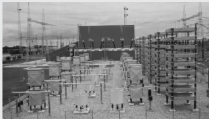
Figure 1 HVDC converter station with ac filters in the foreground and valve hall in the background
