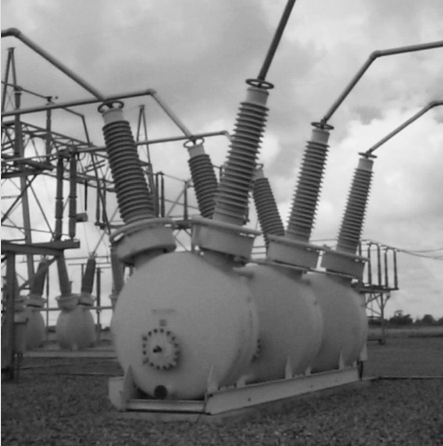
345-kV SF6 circuit breaker installation at Goshen Substation, Idaho Falls, Idaho, USA. This circuit breaker has a continuous current rating of 2000A and an interrupting current rating of 40 kA (Courtesy of PacifiCorp.)
